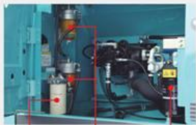
Main fuel filter Pre-fuel filter (with built-in water separators) Engine Oil Filter
